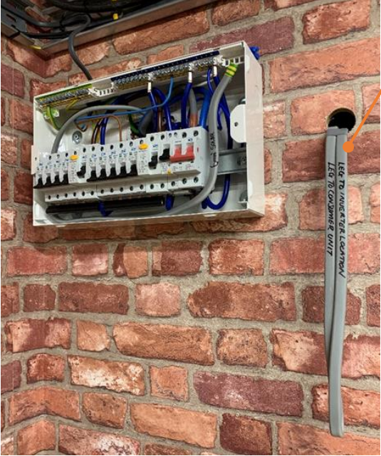
Local loop left for isolator and meter
