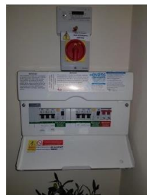
Example 1. Fuse board and isolation switch
