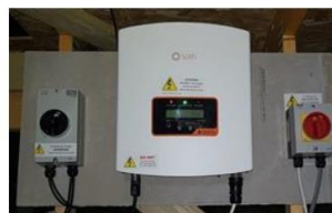
Example 2. - Inverter and isolation switches in loft space
